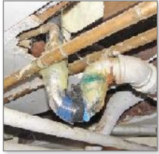
example: Plumbing Code violation
