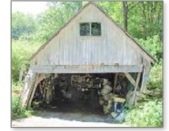
example: Dangerous Structure violation
