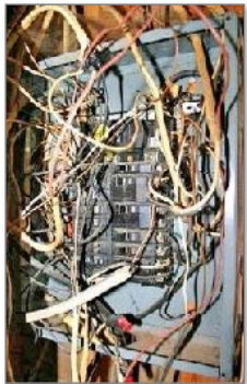
example: Electrical Code violation
