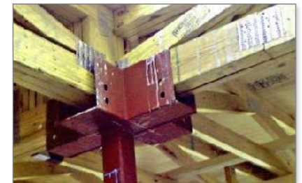
example: Building Code violation
